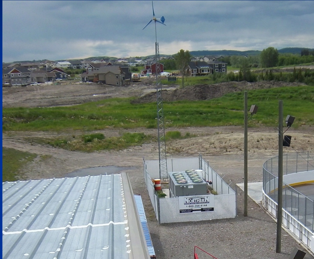
Regular style wind turbine beside the Scott Seaman Sports Rink
