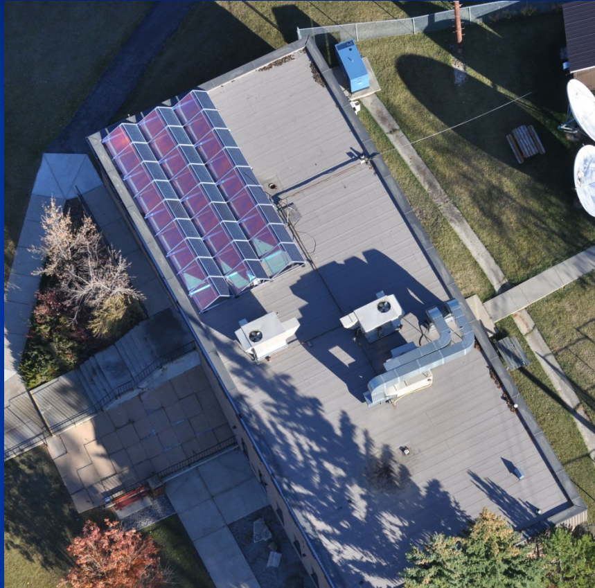
Reflector Solar System on the Black Diamond Town Office
