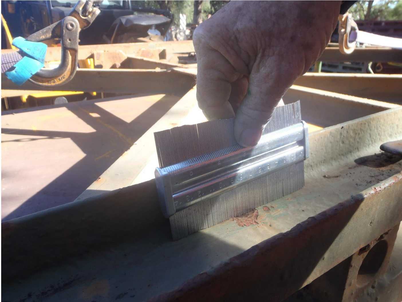
Measuring depth of corrosion
