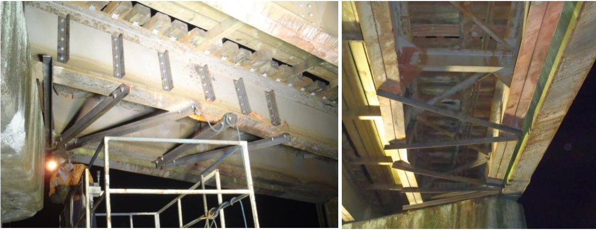
Picture 7 and 8 – Temporary cross bracing and web stiffeners installed (Photo Credit: Cody Young)
