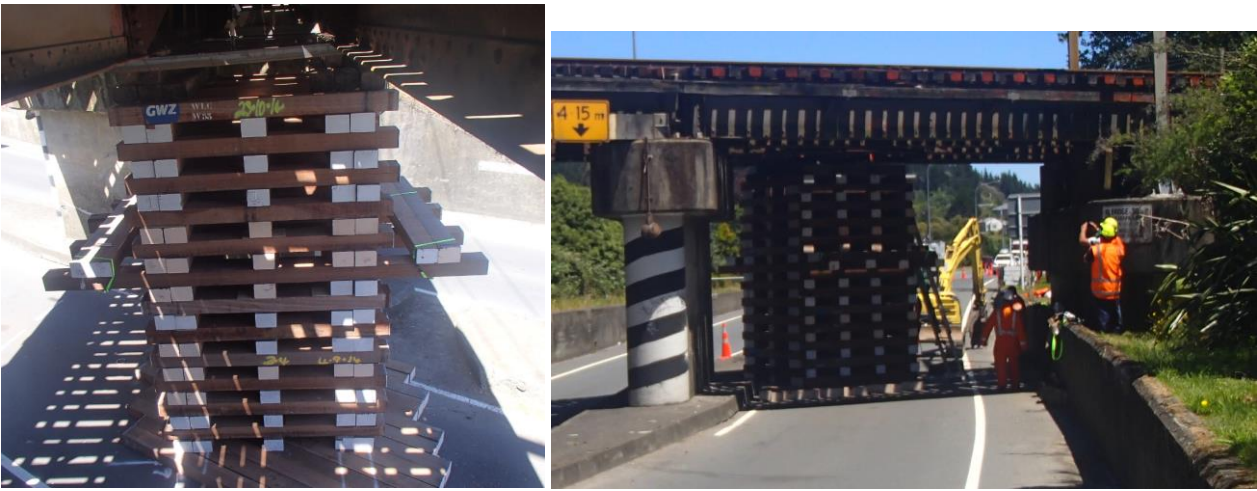
Picture 9 and 10 – The sleeper pigsty installed under the span (Photo Credit: Derek Jansen)
