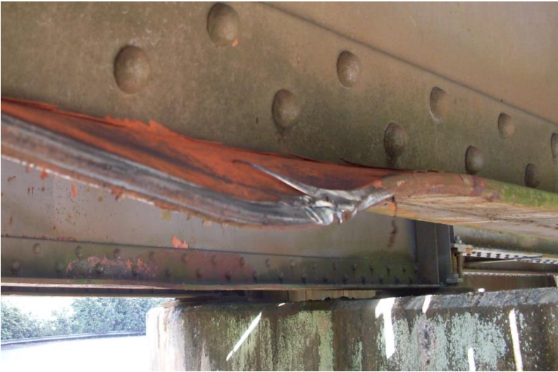
Picture 6 – Approx 60mm tear in bottom flange (Photo Credit: Graham Boorman)
