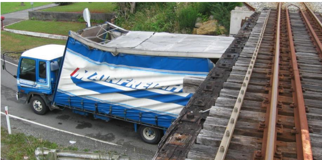
Picture 1 - A typical example of a truck that has come off worse after a bridge impact with little actual damage to the bridge span (Photo Credit: Unknown)
