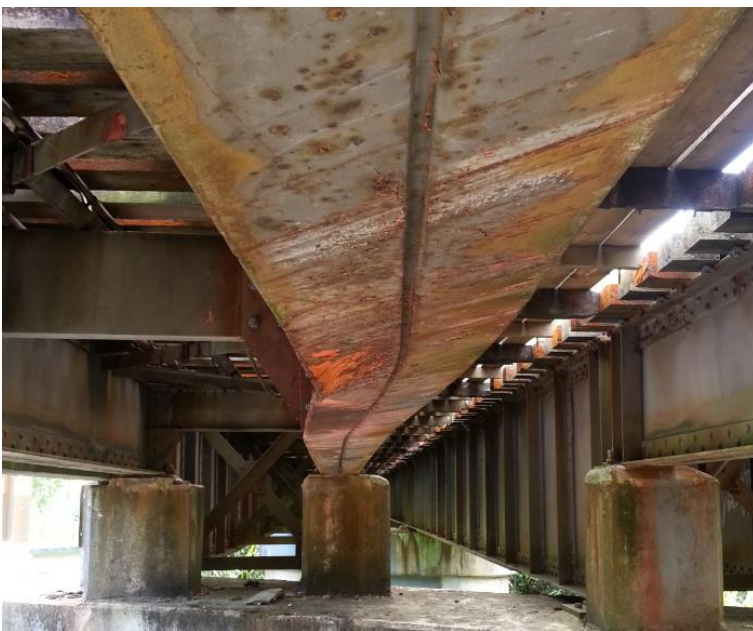
Picture 5 - Side 1 bottom flange global lateral deflection (Photo Credit: Michael Luke)
