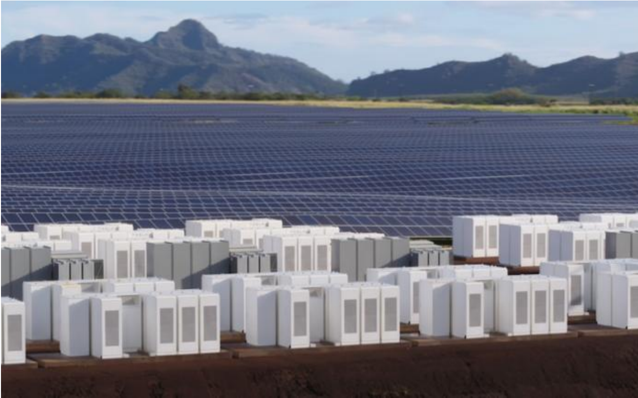
Above Left: Tesla Li-Ion batteries at Kauai solar farm
