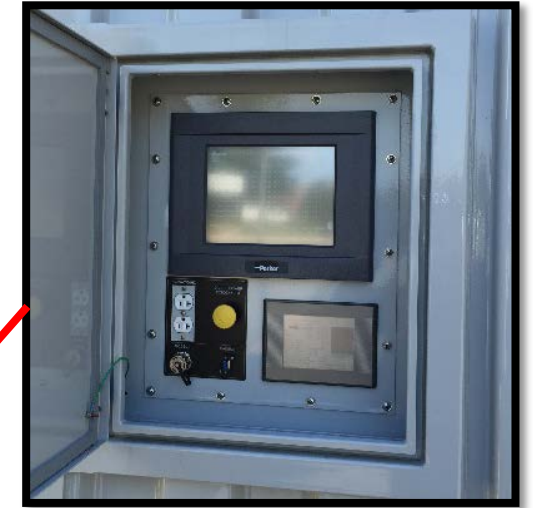
Battery Container HMI
