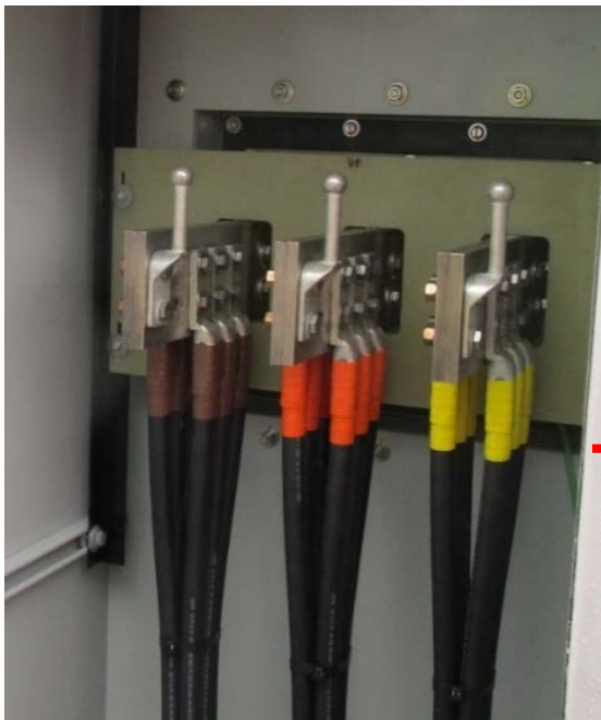
AC Connections and Breaker
