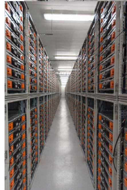
Right: Li-Ion modules in Tehachapi
