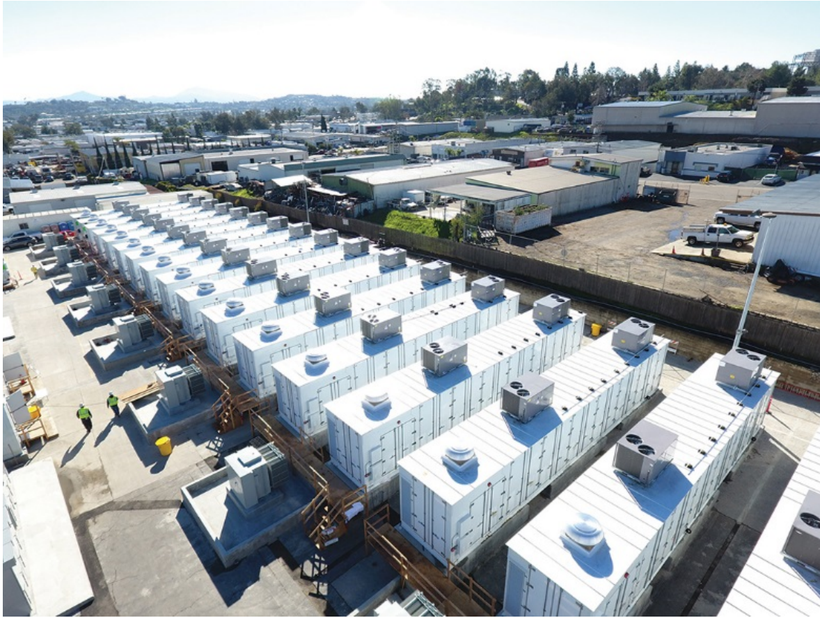
Above Left: SDGE, Escondido 120 MW installation
