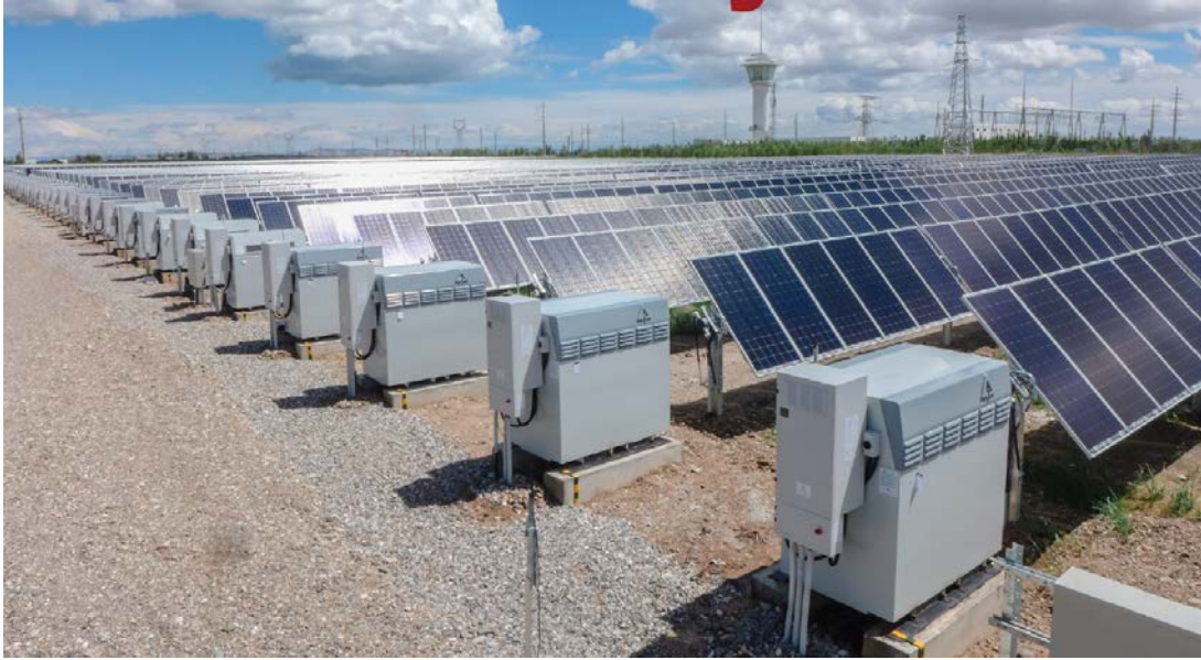
Avalon batteries tied to solar array, 40kW-hr modules
