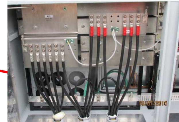
DC Battery Power Connections
